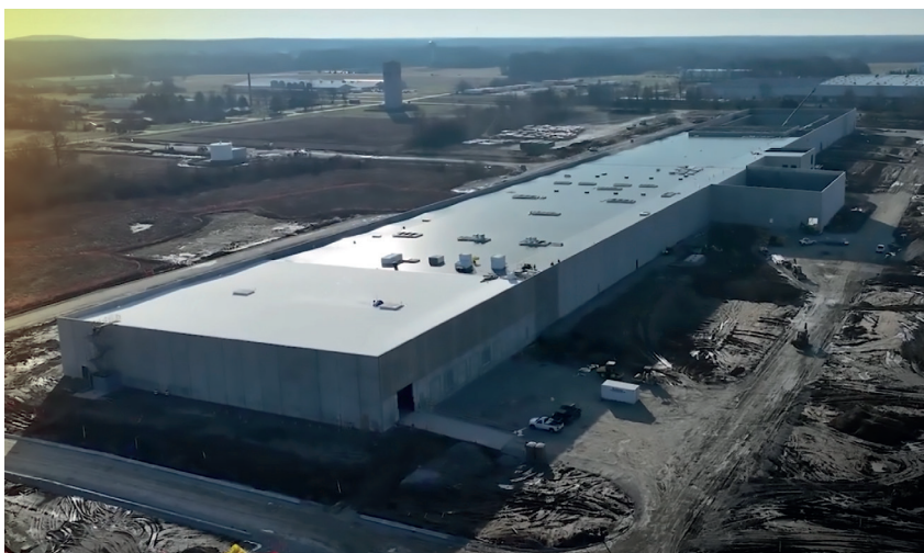
Above: ENTEK broke ground on the Terre Haute facility in September 2023 after scouting for the right location for over a year and construction is well underway (below)
